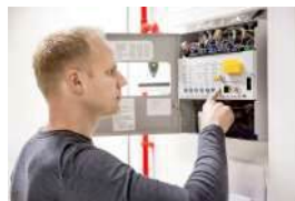
AMC of Fire Alarm System
