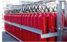
Fire Flooding System
