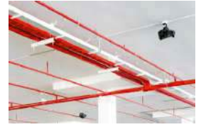
Fire Sprinkler System
