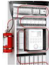
Automatic Fire Suppression System
